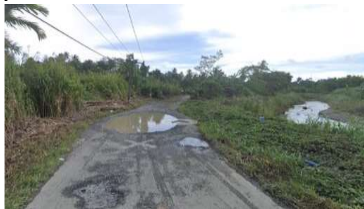
Figure 2. Condition of the road to Pantai Indah Sirombu
